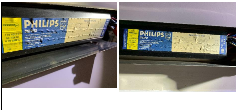
Photo 1 – Philips RQM Lamp Ballasts. Ballast marked as non-PCB's.
